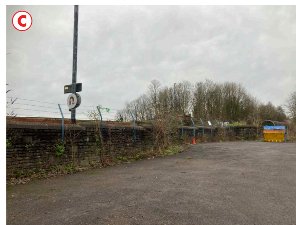
View across site looking south-eastward along rear of Bath Road boundary wall
